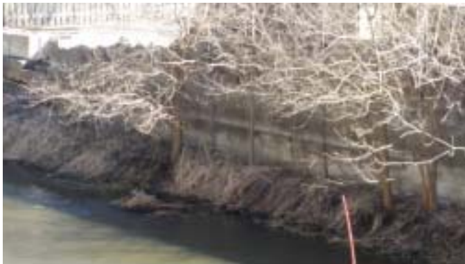
Top of lower concrete wall to remain is approx. 2 feet above the FEMA 10 Year Flood Profile (which we are using for the ordinary high water mark
